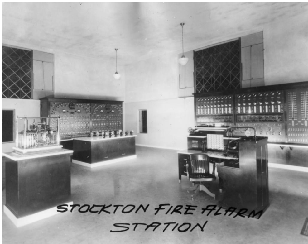
Photo 6: Control and Instrument Room of the Fire Alarm Station (Haggin Museum)
